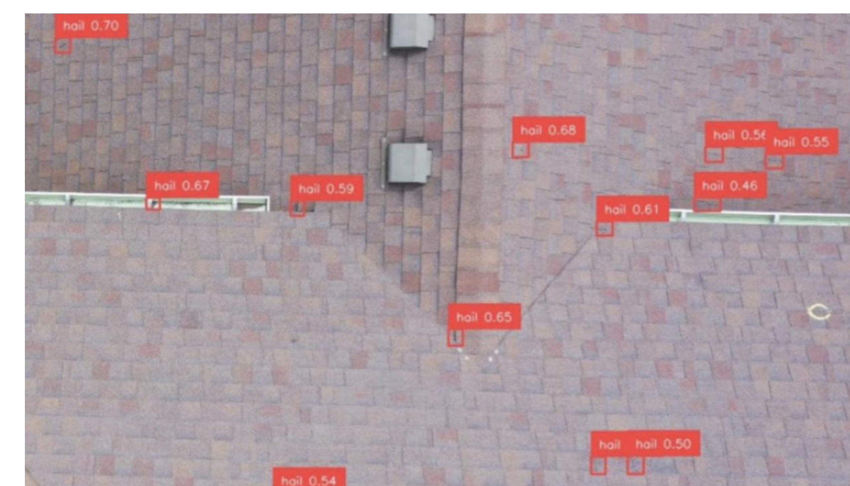
Figure 3. Top-down UAV image of a residential roof with hail damage detections from our model, shown as red bounding boxes with confidence scores [3]
