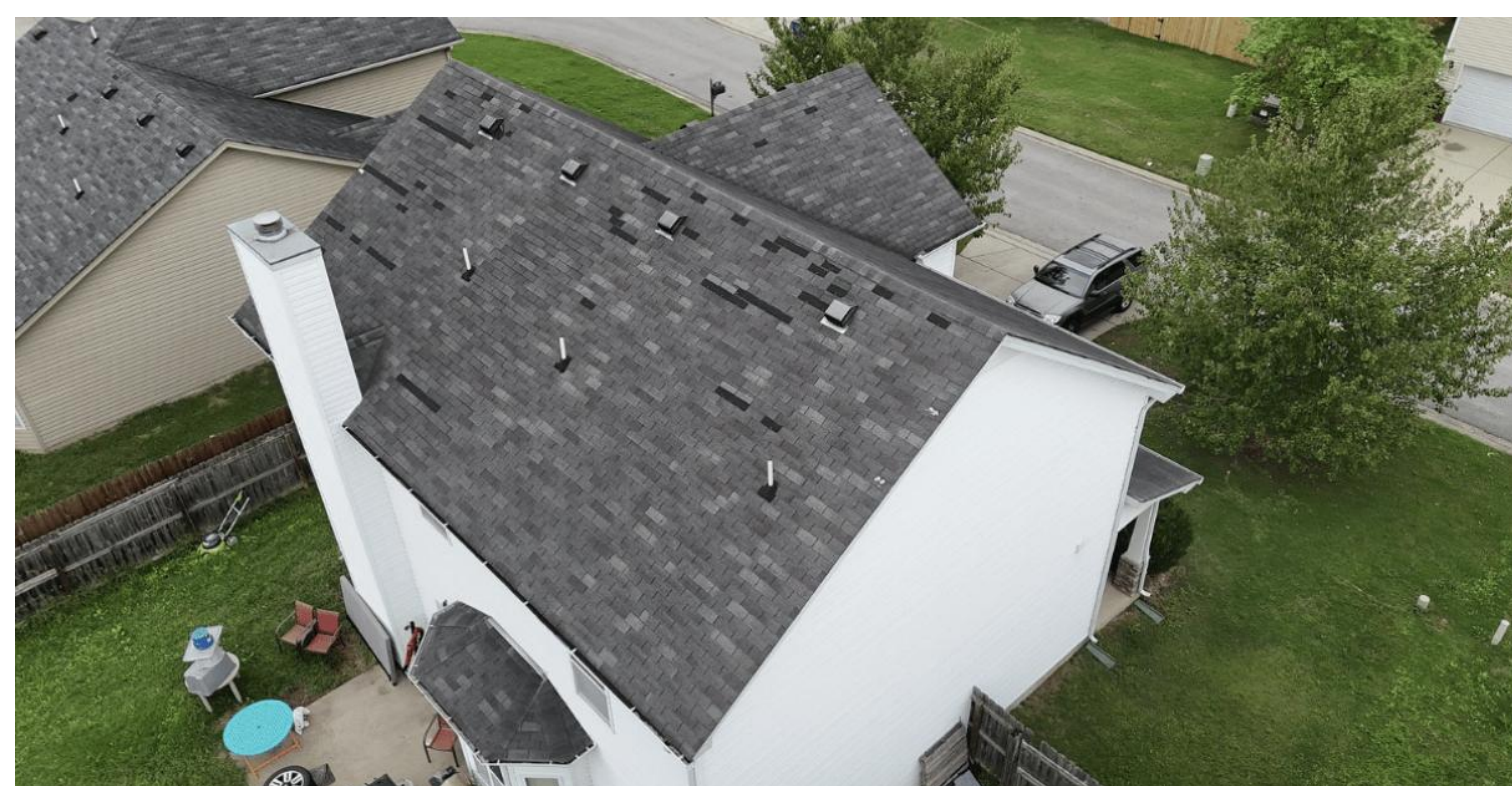
Figure 1. UAV-captured image of a residential roof showing missing shingles caused by wind damage. [5]
