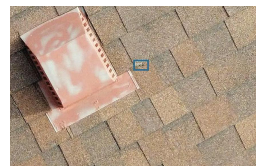
Figure 10. AI Hail Damage Detection
